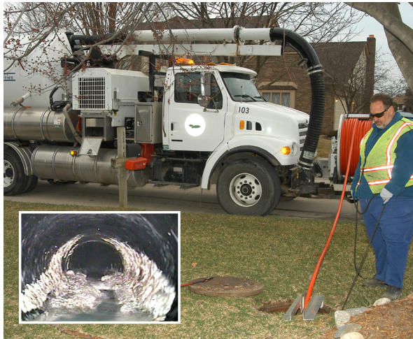
FOG build-up in sewer pipes (inset photo) requires local public works staff to go to the site and remove the blockage. The extra maintenance required to clean the sewer comes at a cost to all sewer system users.
